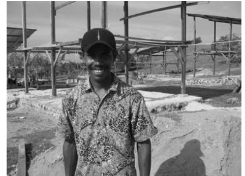
Dahlan, 37, was chosen as both head and housing coordinator of his sub-village of Lamreh. The IDPs have agreed among themselves on a uniform type and size of house that will be rebuilt for each family in the village. Abdi R. Tarigan, ACT.
